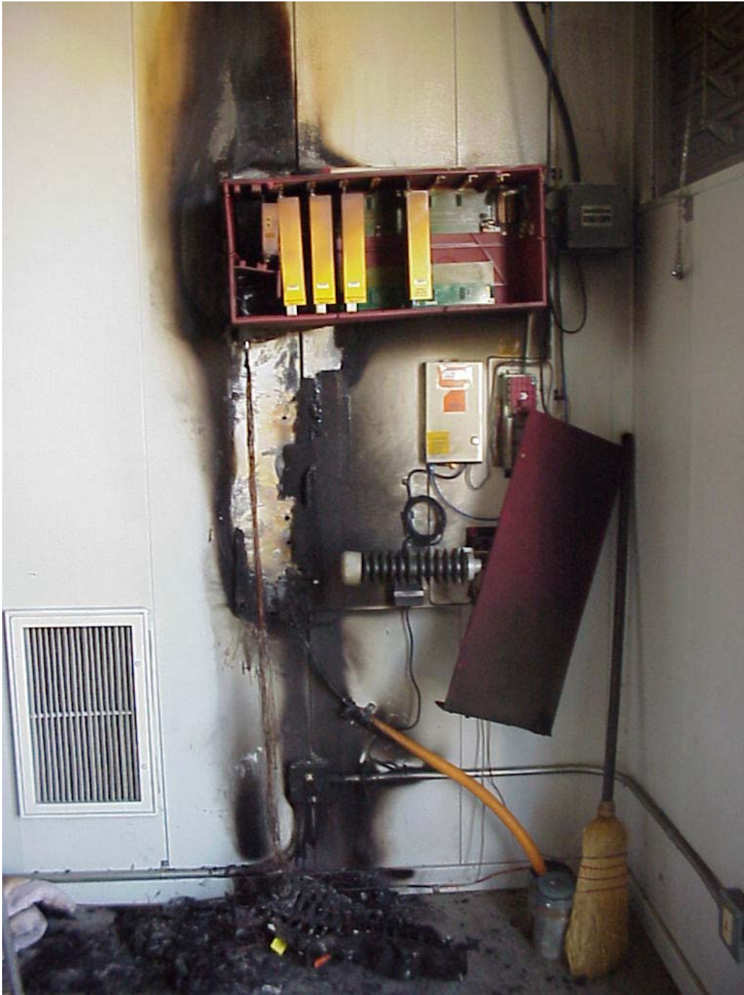
The above location is a Power Plant in southern California. It has yet to be determined what additional damage has occurred since this fault happened only a few days ago on March 23 rd 2002.
